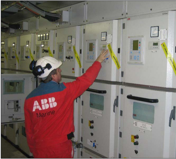
Picture 2: Medium-voltage switchgear monitored by fixed pyrometers
