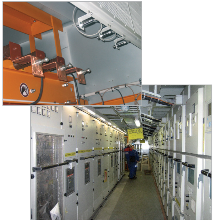
Typical monitoring locations at points of contact; Medium-voltage switchgear monitored by fixed pyrometers
